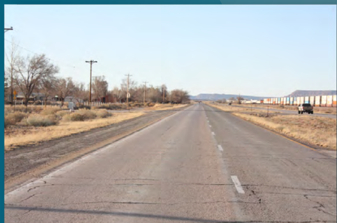
Narrow Roadway Shoulders
