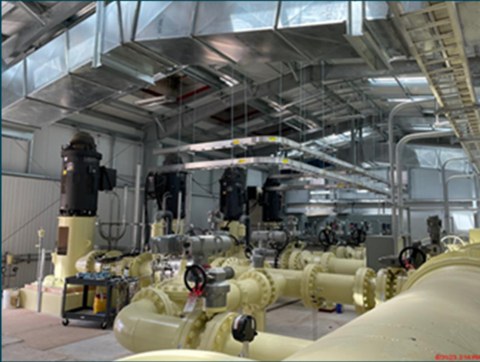
Pumping Plant 4 Interior Pump Room
