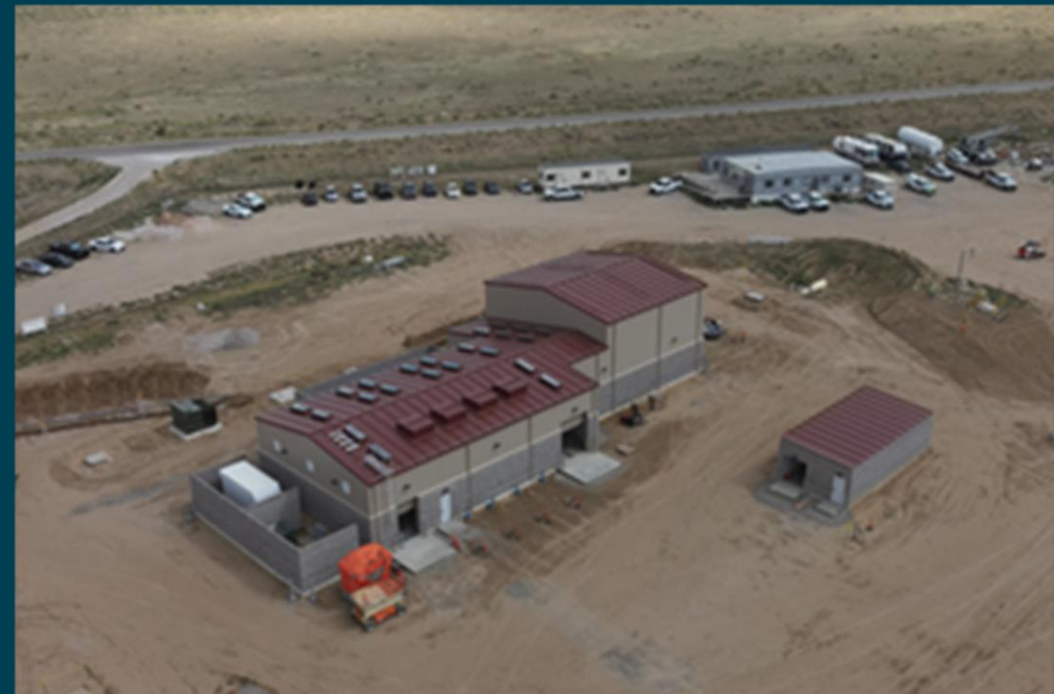
Pumping Plant 7 Aerial Photo
