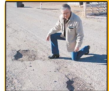
Grants Mayor Joe Murrietta looks over some major road damage on Estancia Street in Grants. A recent GRT increase will net the City approximately $400,000
